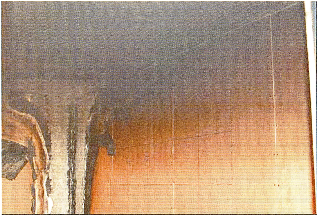
Figure B-8. End of Test; View of Right Wall at Ceiling.
